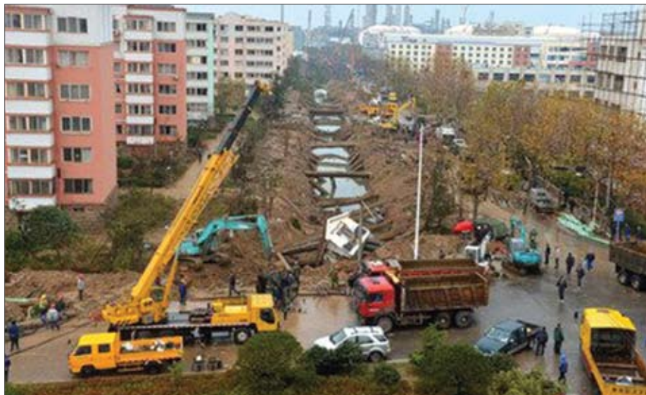
Figure 4. Gas line explosion in Qingdao
